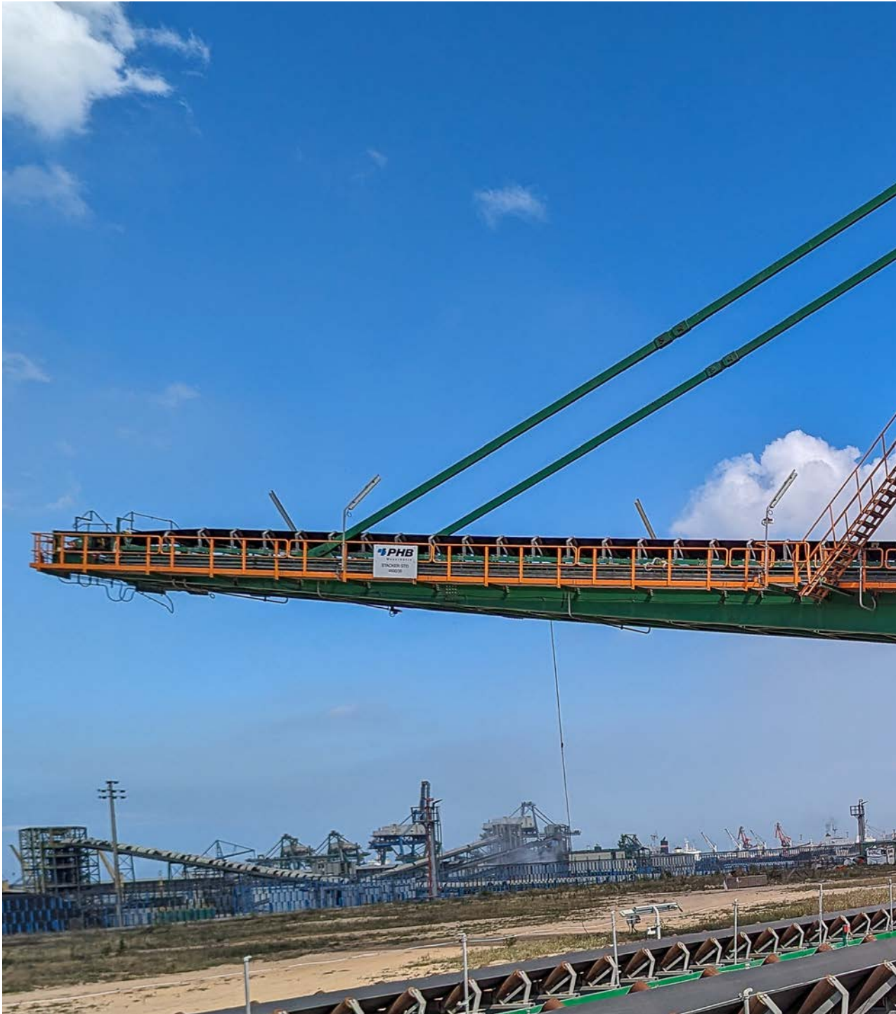
COAL HANDLING SYSTEM. JORF LASFAR THERMOPOWER PLANT (MOROCCO)
