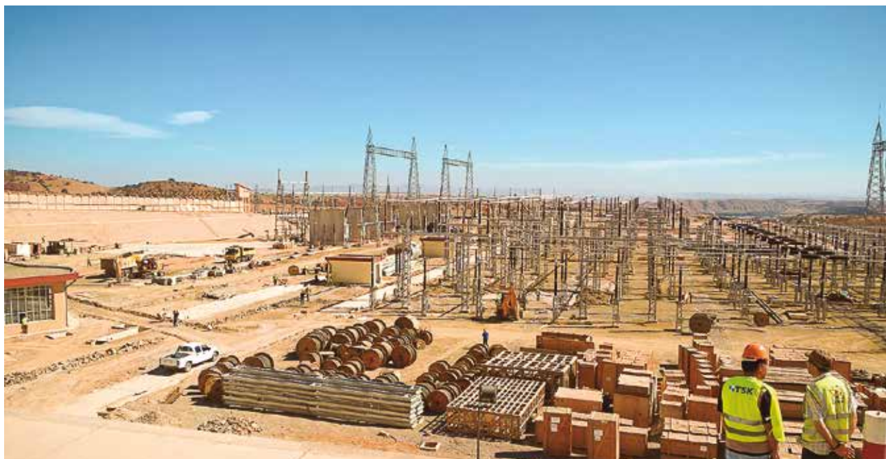
400 kV Substation Aih Fateh (Algeria)
