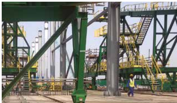
Sulfur handling system and ship loading facility Jazan Refinery (Saudi Arabia)
