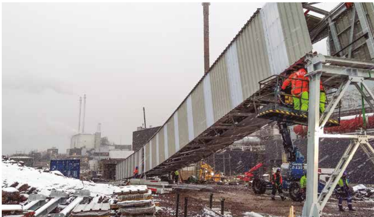
Complete handling system for coke and asphaltene. KILPILAHTI Power Plant (Finland)
