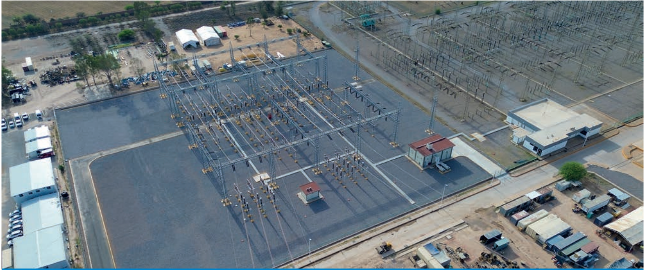
230KV SUBSTATION. SAN LUIS DE POTOSI 450 MW COMBINED CYCLE POWER PLANT (MEXICO)
